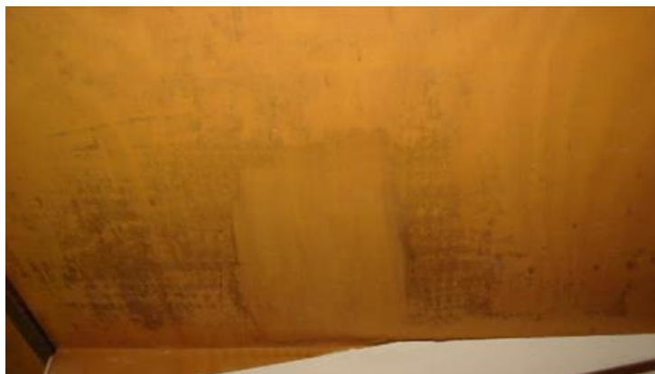
Typical example of surface mould
