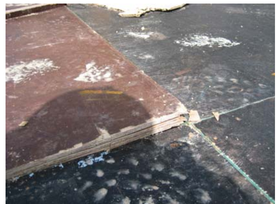
On-site comparisons: In the Sutherland test case, the black material, which is EWPAAs certified, has performed well. The brown Chinese material has lifted and has delaminated.
