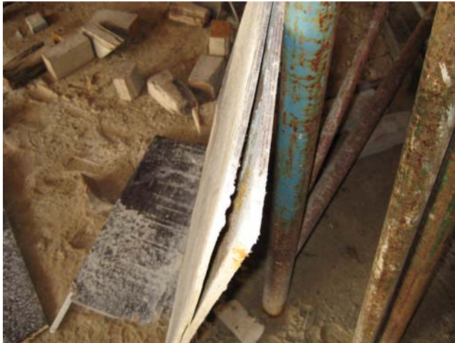
Image shows severe delamination of the central glue line on the condemned formply at the Sydney construction site.
